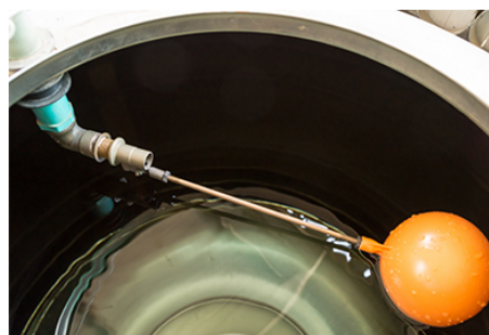
Level control float switch
